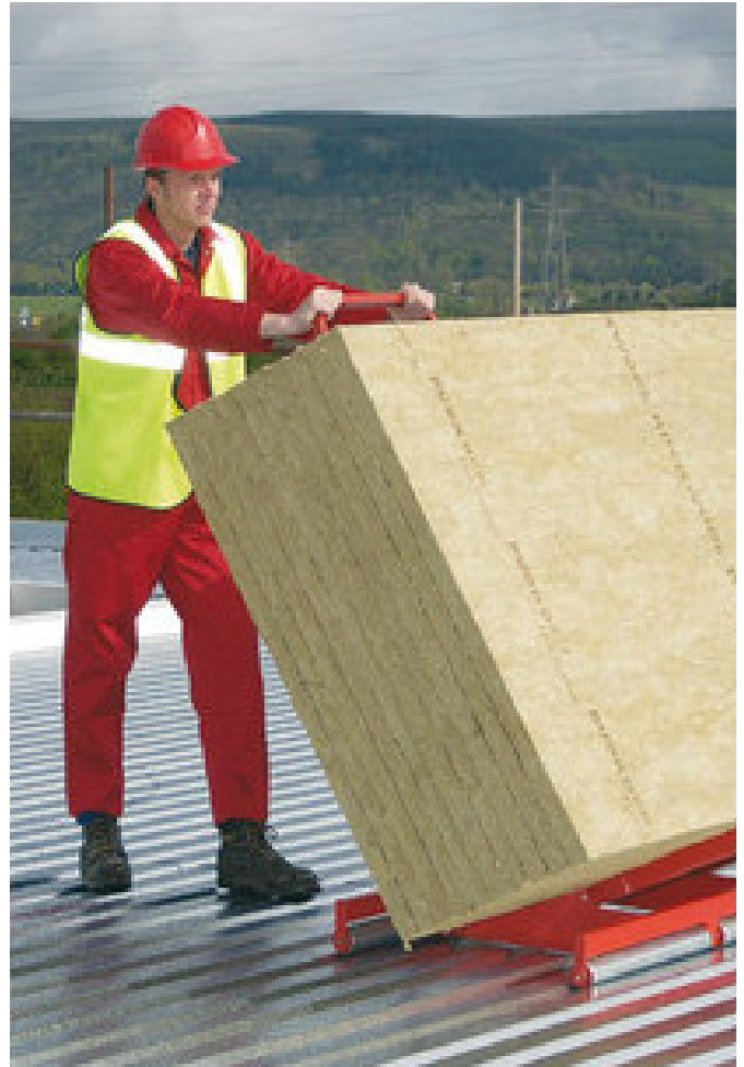
Use of the ROCKWOOL® Rock Roller trolley allows fast and easy movement of boards across the roof decking.
